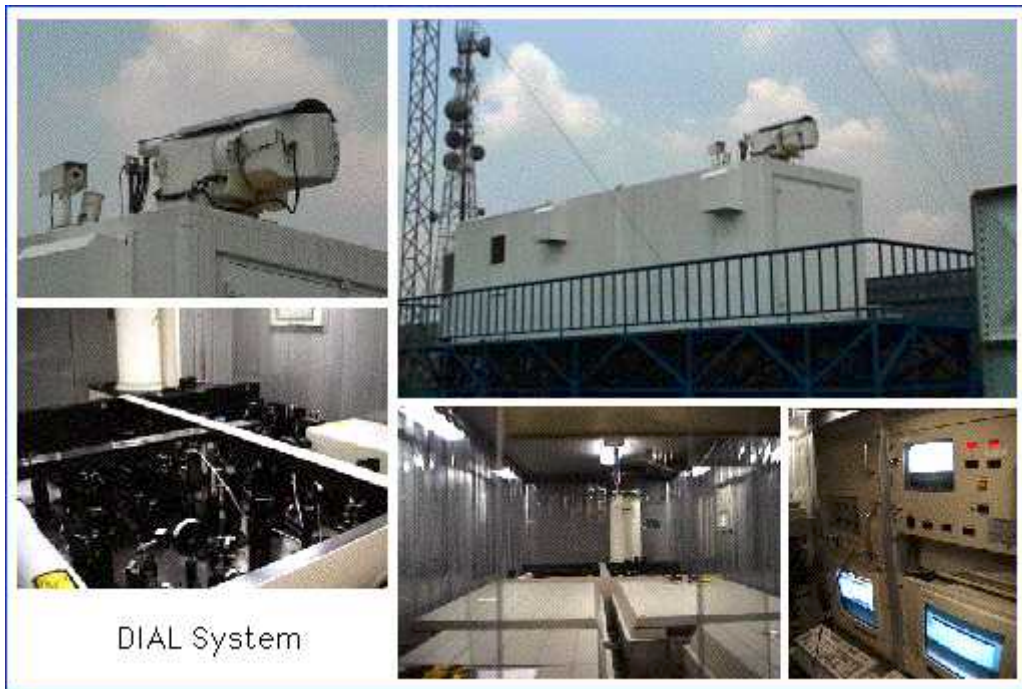
DIAL installed on the top of the LIPI Headquarters Building at Gatot Subroto Street (PINANDITO et al. , 1998)
