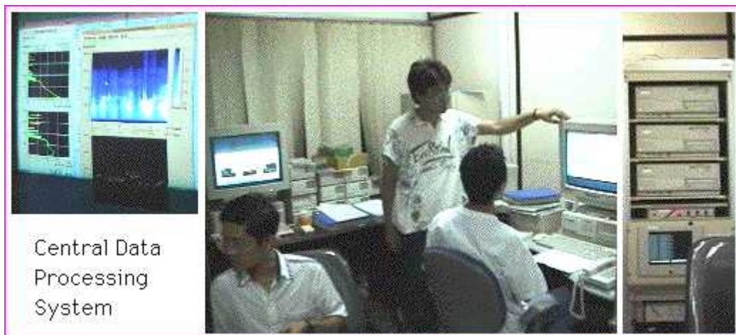
Central Data Processing System installed in the LIPI Headquarters Building at Gatot Subroto Street (PINANDITO et al. , 1998)
